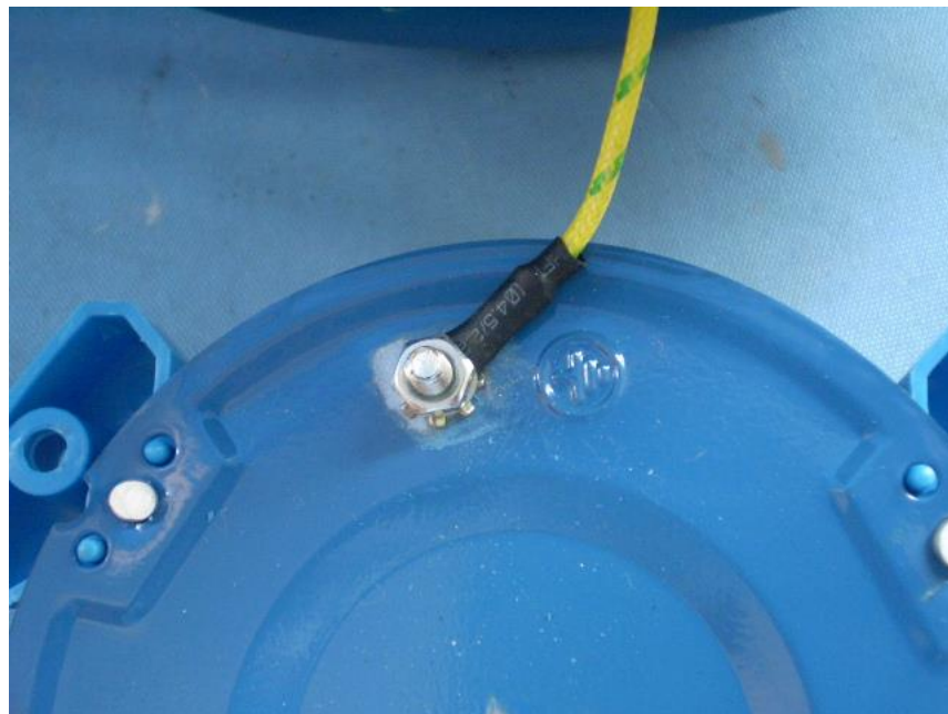
Earthing for RCW-2
