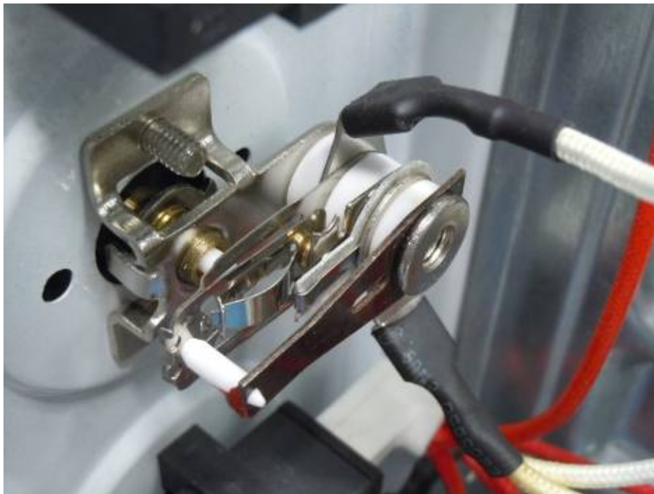
Overall view of thermostat
