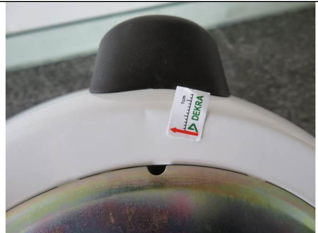
248. Slight dent mark on housing
